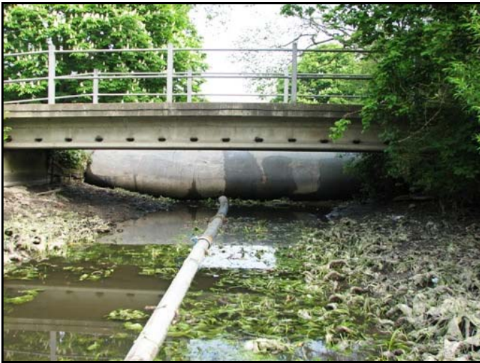
Picture 2: Downstream of the AquaDam in the working area on the River Colne, West London, showing one of the bypass pipes running under the dam (NE Thames Operations Delivery)
