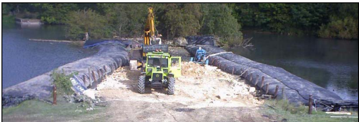
Picture 4: Two 40m AquaDams installed in a lake at an English stately home (Courtesy of Albion Water Structures Limited)
