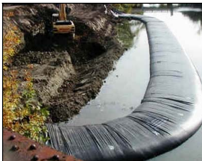
Picture 1: AquaDam installed around the working area to prevent materials entering a live watercourse (Courtesy of Albion Water Structures Limited)
